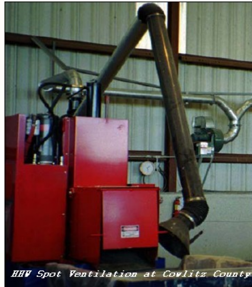
Local Ventilation connected to Hepa Filter
